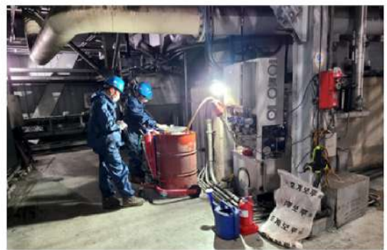
4. HPU Oil Drain
