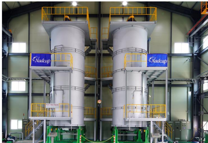
Solution Furnace -Vertical 1.5m(Ø) x 5m(H)
